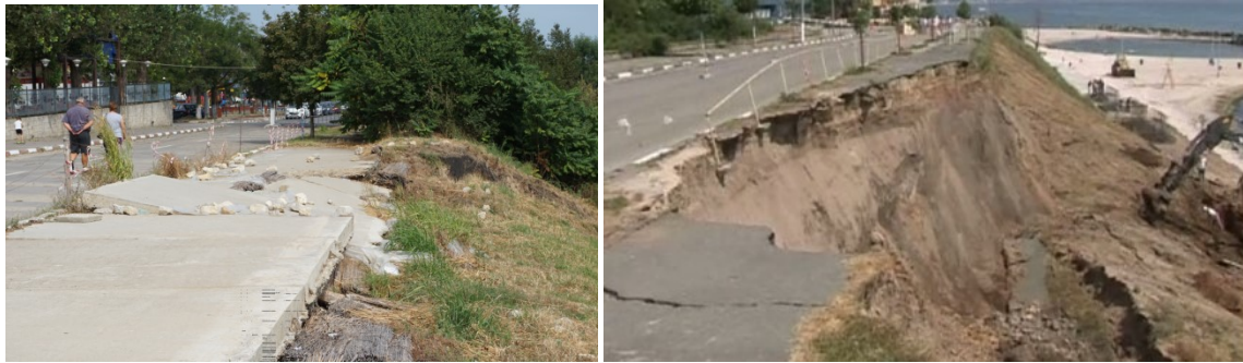
Fig. 3.5. c and d - Landslides under the promenade alley/sidewalk Eforie South
